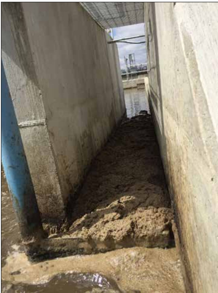
Figure 3: Nitrate Recycle Gate Closed
