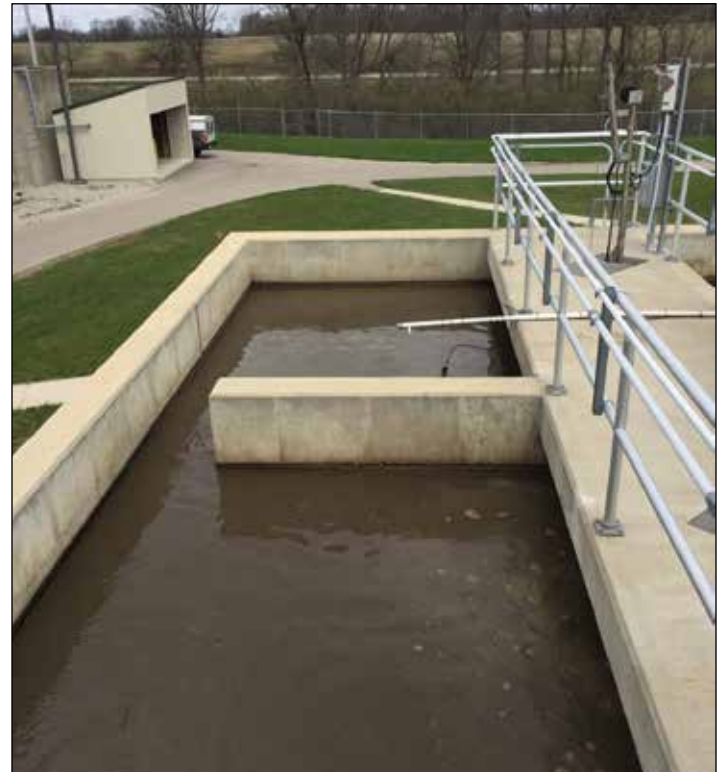
Figure 2: Anaerobic Tanks (Mixers ON)
